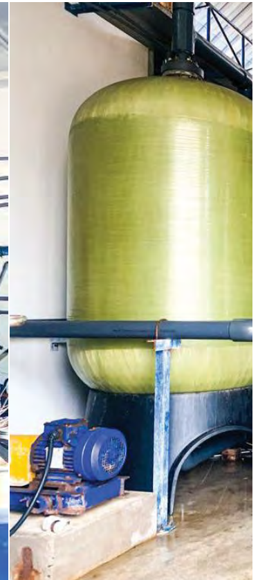
Water pump in SWRO Building Source: Jakarta Water Resources Department
