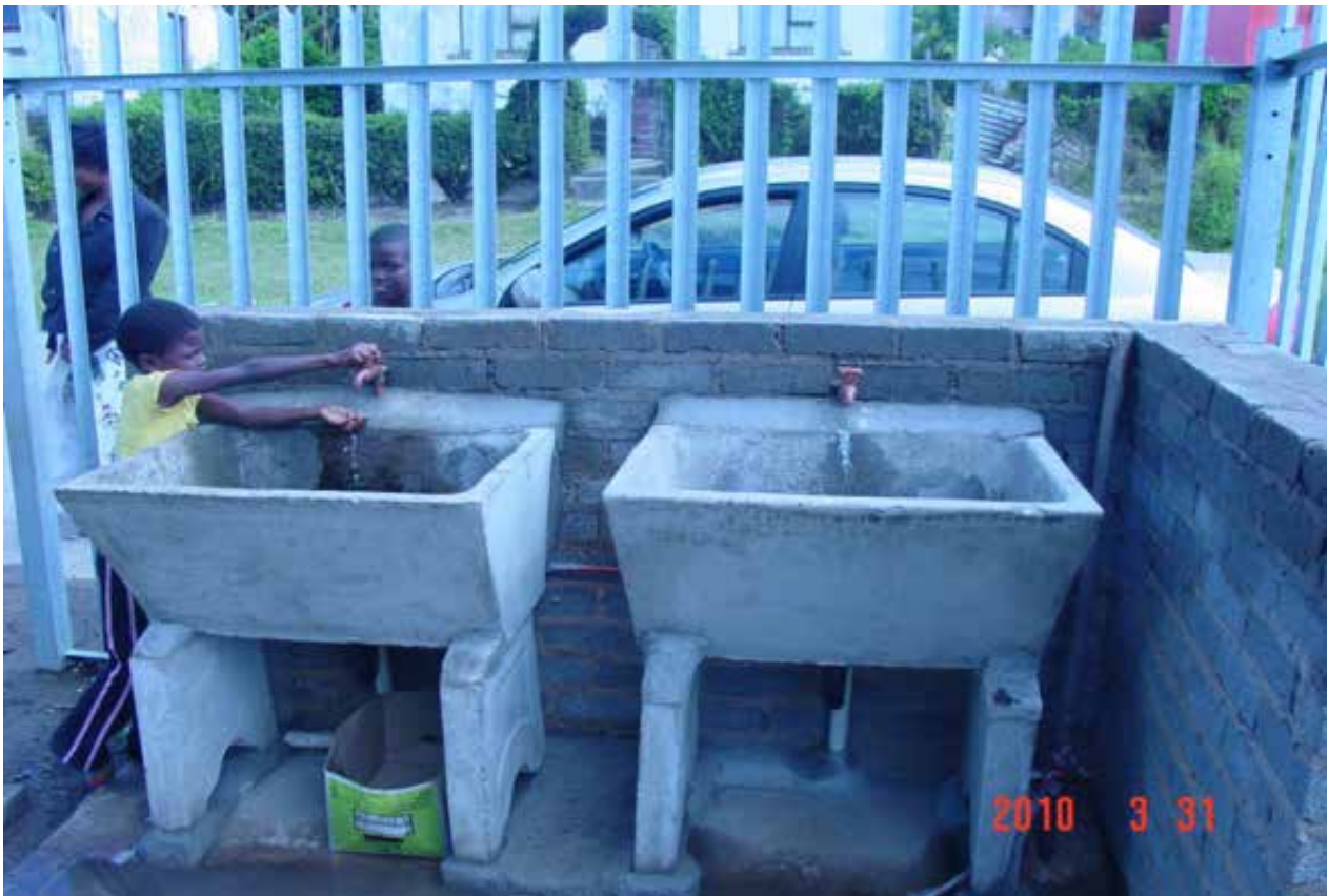
Plate 5: Communal water & facilities installed in informal settlements
