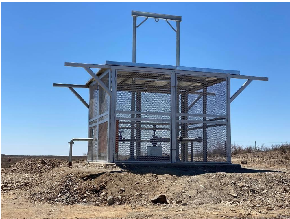
Typical Borehole Pump Station at Romanskolk Wellfield
