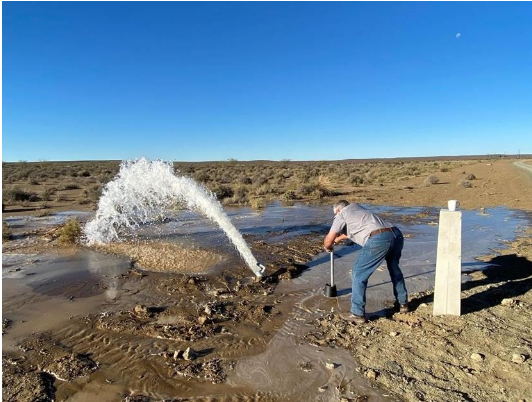
Operation of a scour valve on the Romanskolk to Brandvlei
