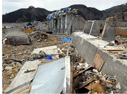
Kamaishi-port (Broken seawalls)
